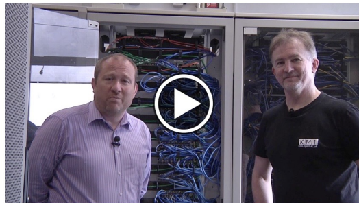
Movie 5.1 Demonstration of a server room.
