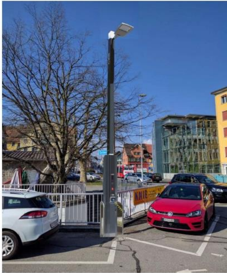
Smart Lighting Pole, Wädenswil, Switzerland
