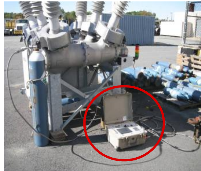
Gas analysis on a DTB, V. Williams, Company EMT
