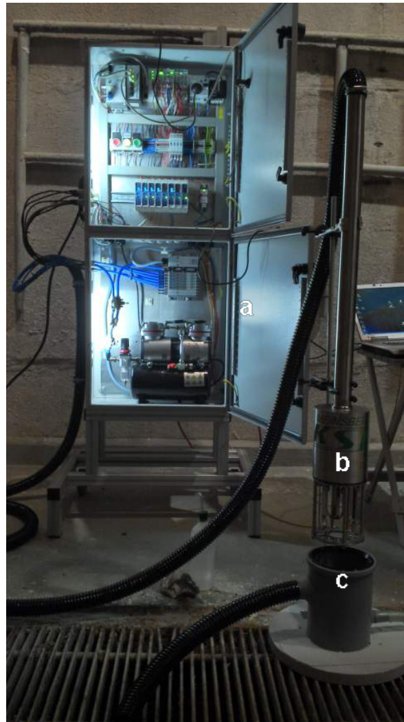
Measuring system for the monitoring of process water, consisting of control box (a), measuring lance (b) and measuring barrel (c)
